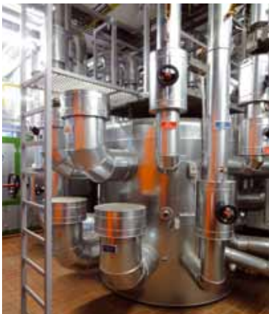
ZORTSTRÖM in Heizzentrale
